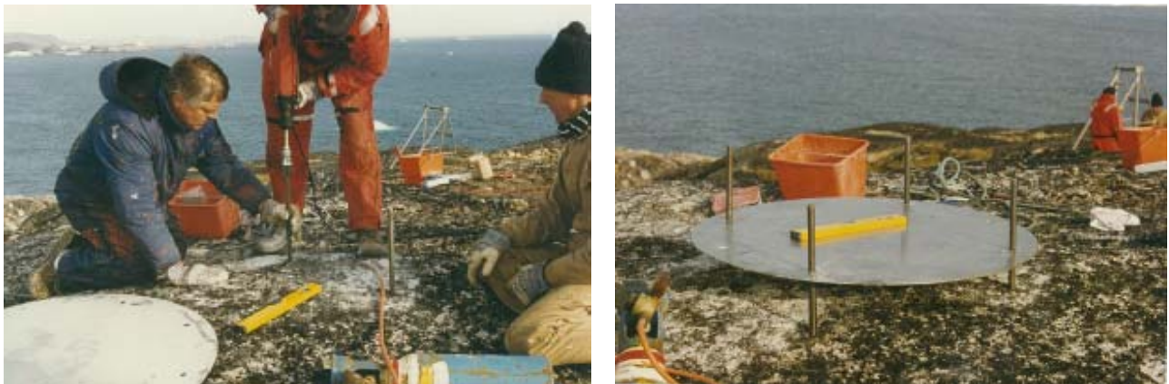
Figure 3 Examples of a simple foundation which is preferred in Polar Regions to ensure a swift installation and to reduce the use of heavy equipment and large quantities of materials.
